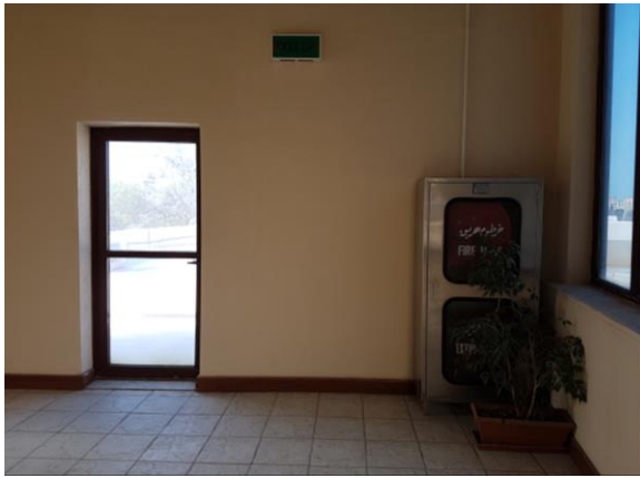
Fig. 5: Fire hose station
