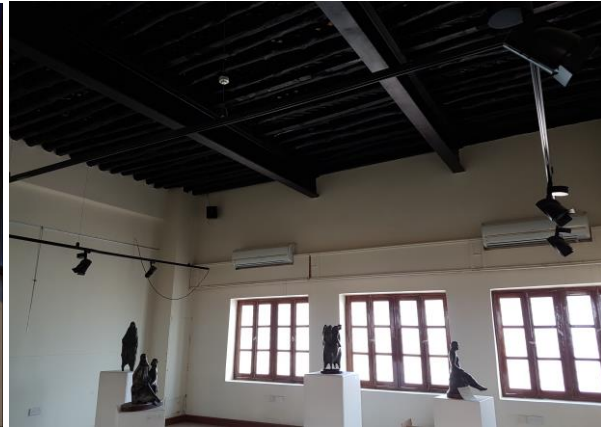
Fig. 6: Air-conditioners and windows
